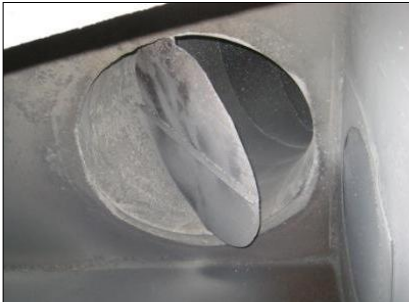
Figure 7.6 Exhaust ducts damper of furnace flue and fume gases
