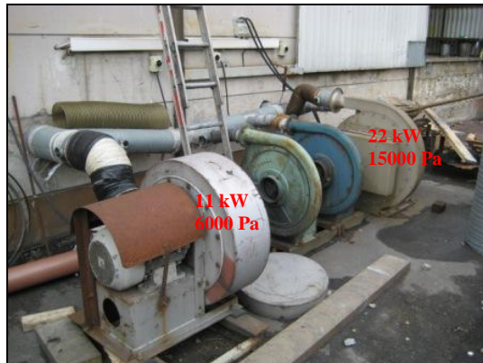
Figure 7.9 Combustion air blowers
